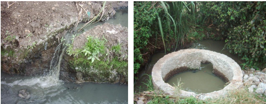
Figure 4.5: Photographs showing sewer burst and tampered manholes
