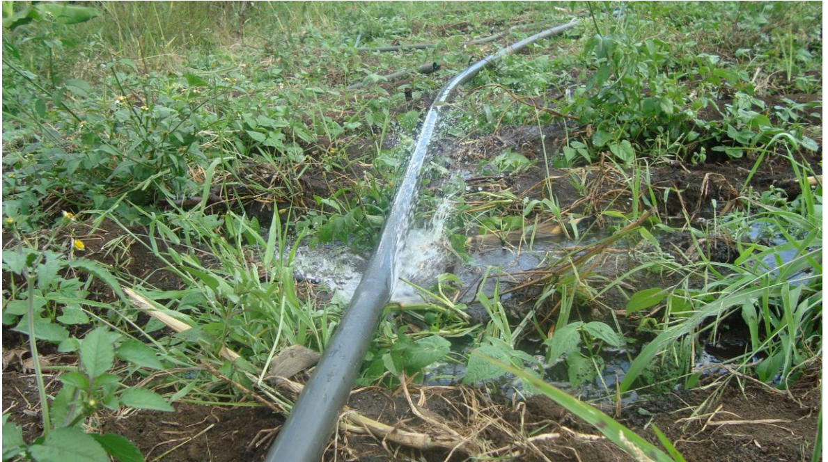
Plate 7.5. Conveyance loss in a leaking Pipe.
