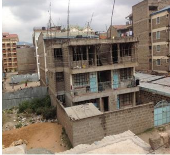
Figure 2.2: Construction of flats in Umoja Innercore estate, Nairobi. Notice that lower floors have been occupied and the building is incomplete
