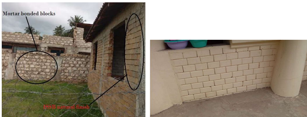
(a) Wall appearance of mortar bonded blocks and ISSB (b) ISSB natural key on the surface
