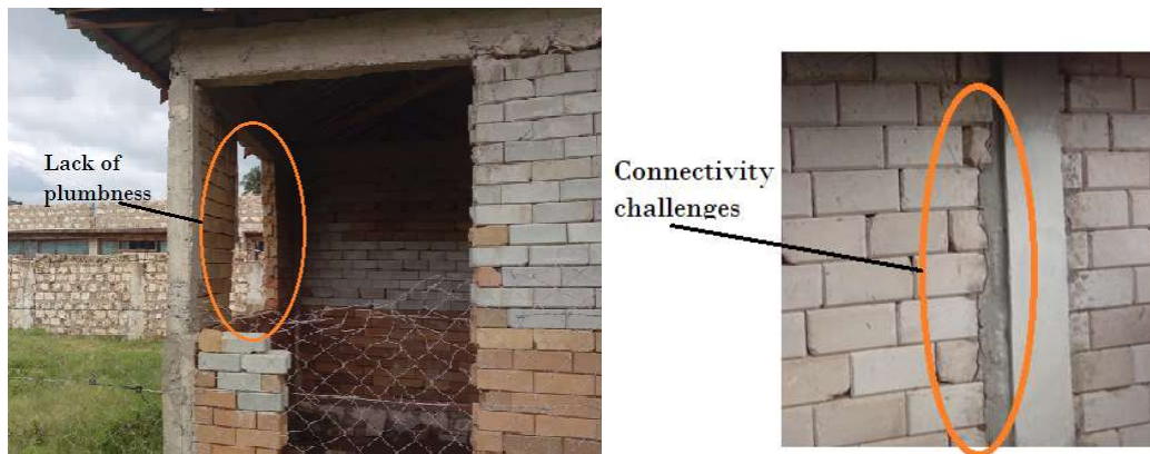
(a) Challenges of wall plumbness (b) Connectivity between blocks and column
