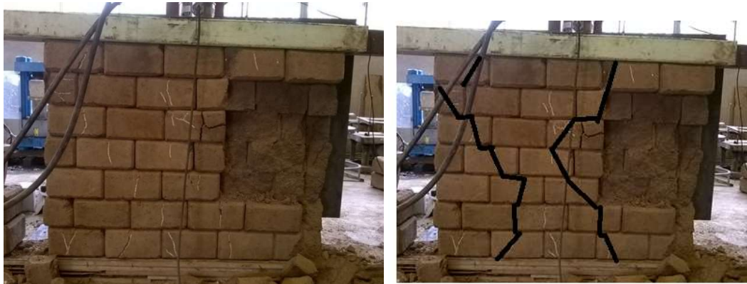
(a) Face cracks on LSW1 panel
