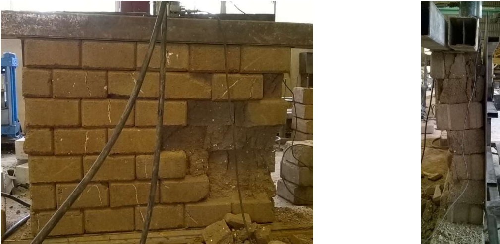
(a) Wall failure and crack pattern at face
