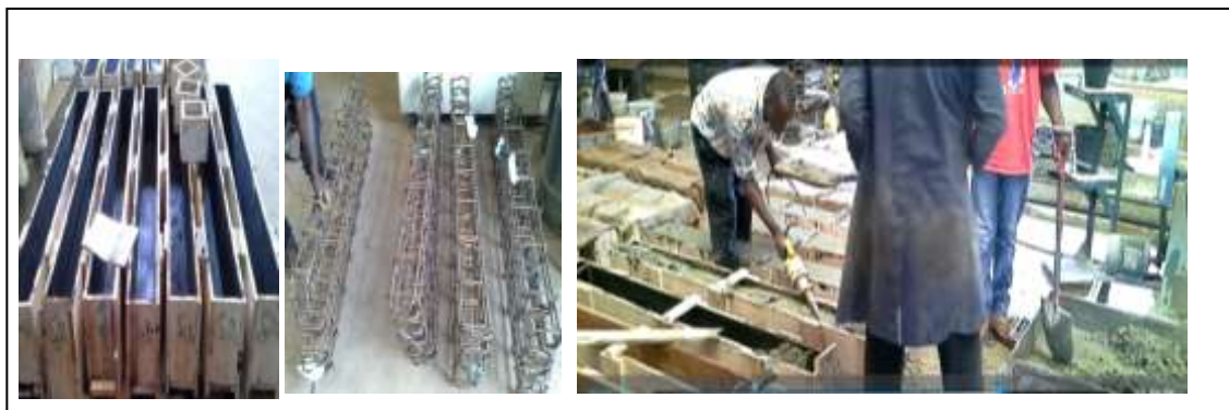
( a ) Beam molds ( b ) Beam steel cages ( c ) Casting of concrete in beam molds
