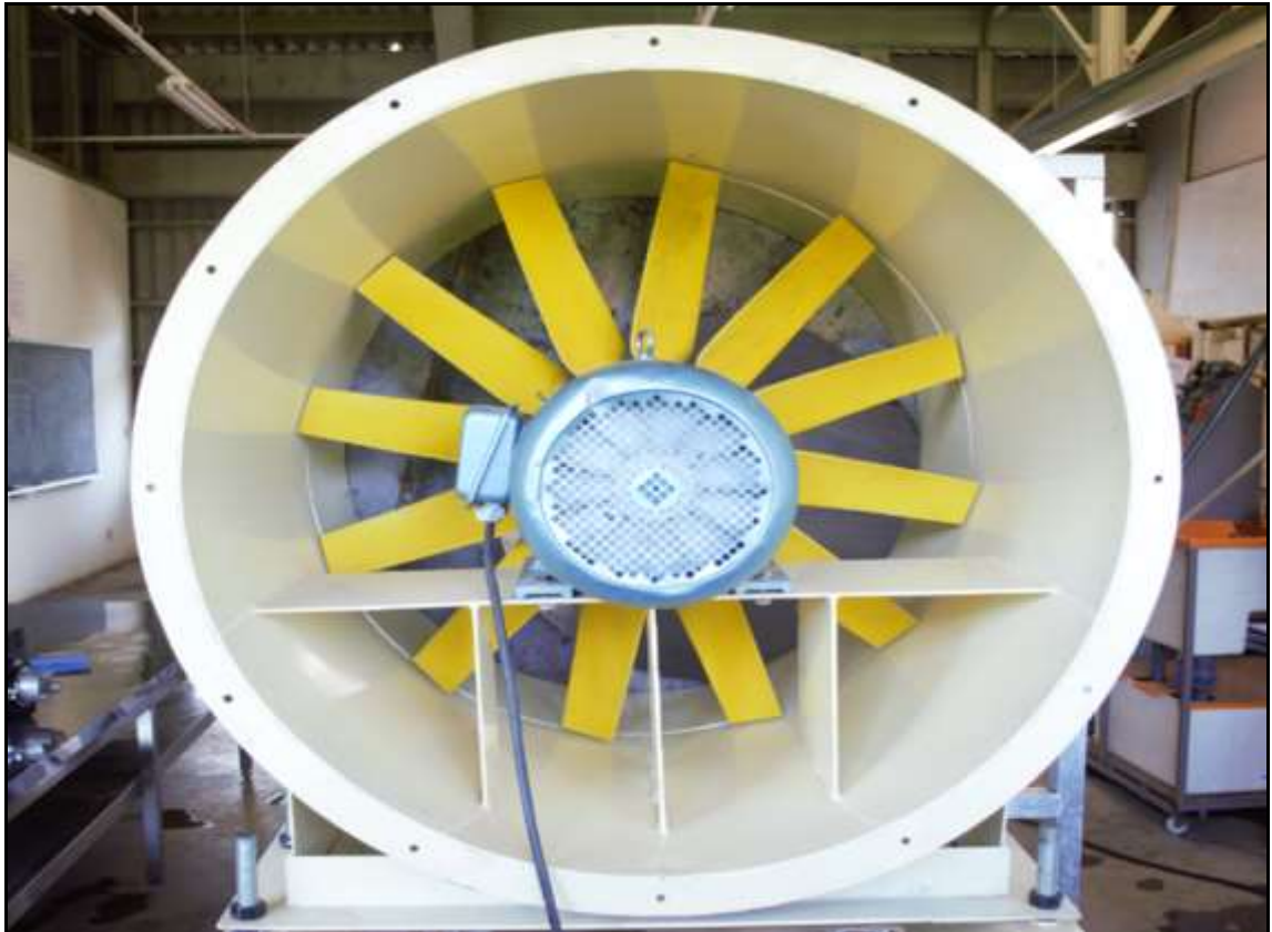
Figure 3.2: Axial suction fan located at the end of the tunnel section
