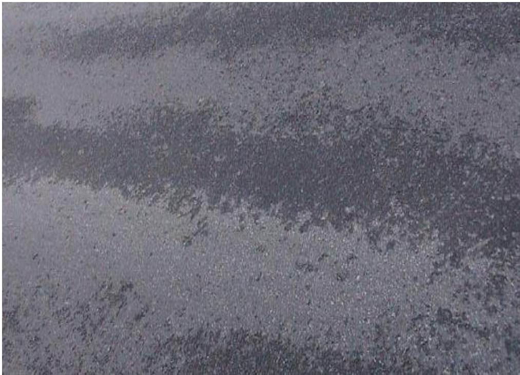
Figure 2.11: Water bleeding (Kamiti road)
