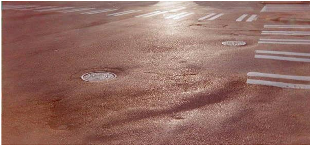
Figure 2.4: Pavement shoving (Isiolo town)
