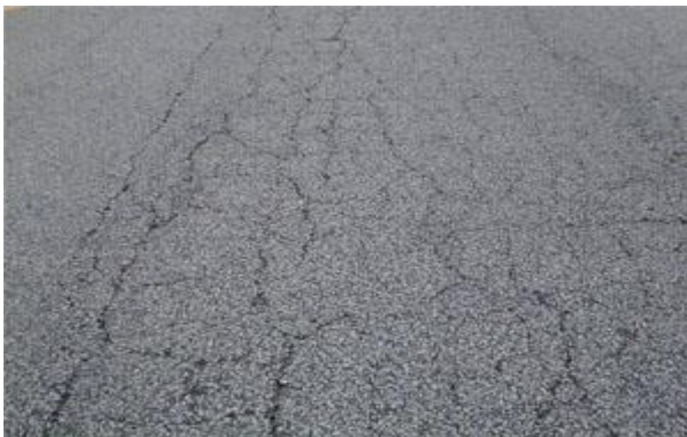
Figure 2.2: Pavement cracking (Muriri-Isiolo road)
