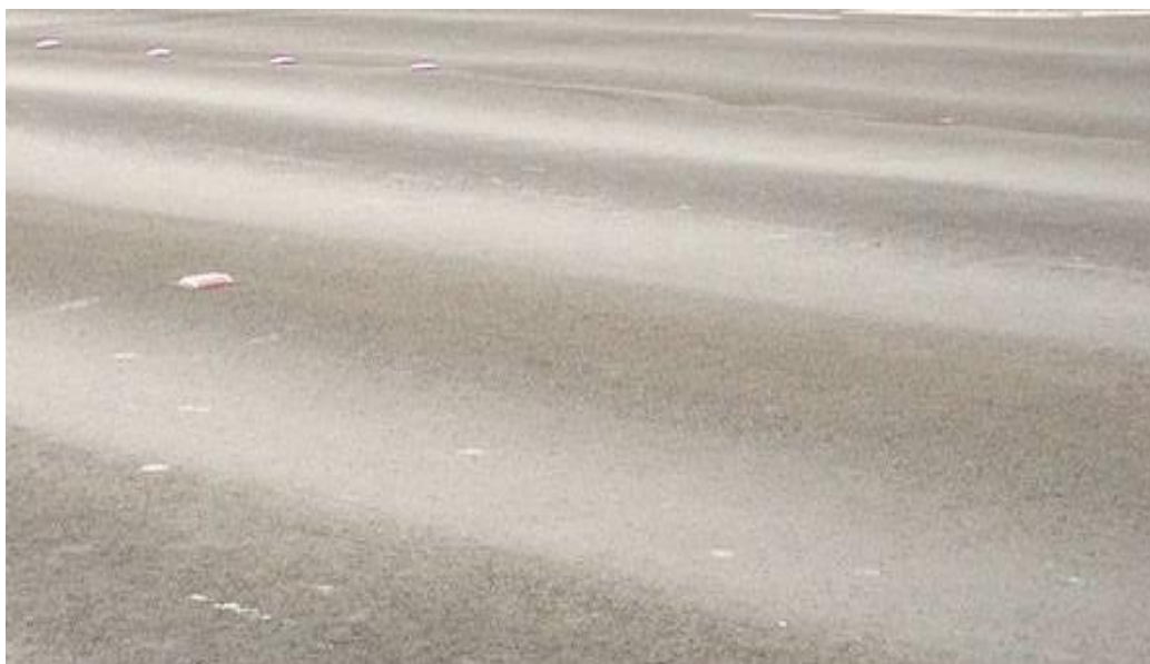
Figure 2.9: Shallow pavement rutting (Meru-Maua road)
