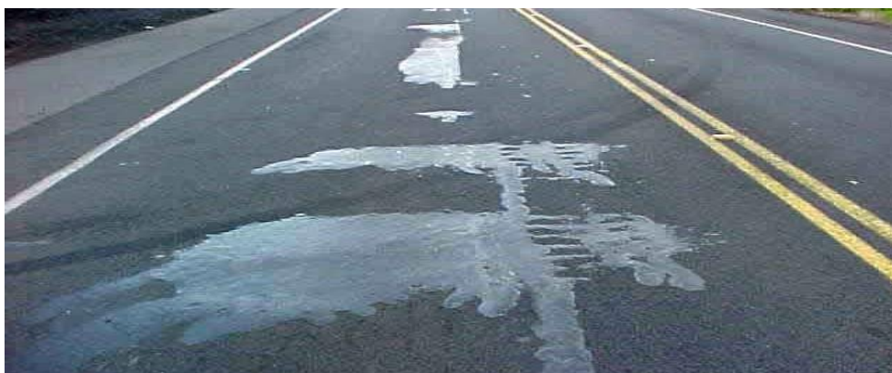
Figure 2.3: Pavement bleeding (Meru-Maua road)
