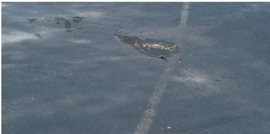
Figure 2.5: Pavement depression (Muriri-Isiolo road)
