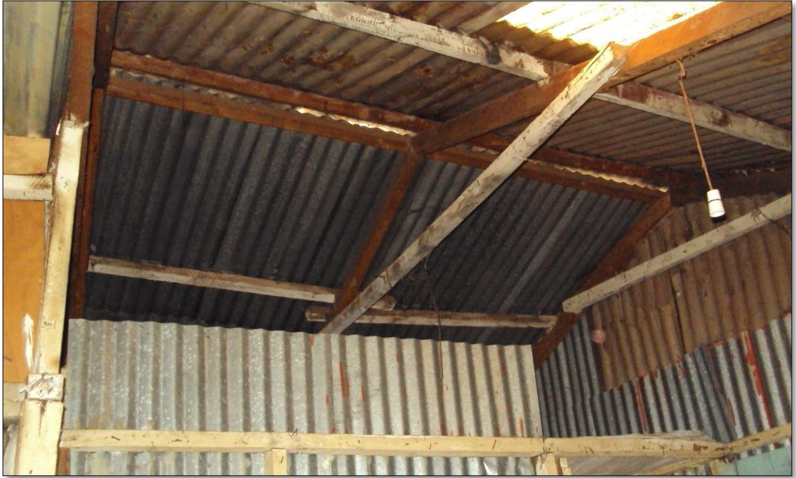
The gable roof structure as for House A and B as seen from inside house A inner room
