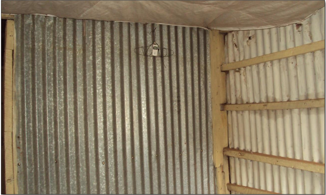
Data logger 2 was set on central partition wall of outer room, House A
