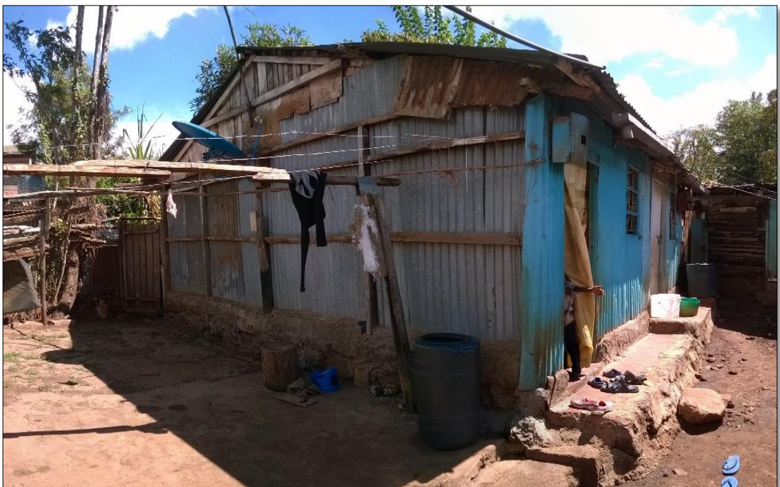
House A and B are made of unlined sheet metal on timber framing
