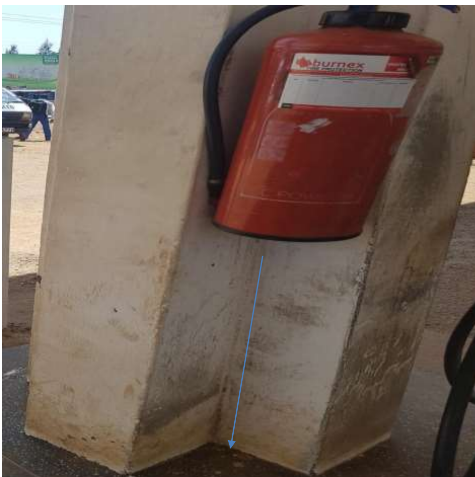
Plate 4.1: Recommended 60cm Height of Portable Extinguishers
