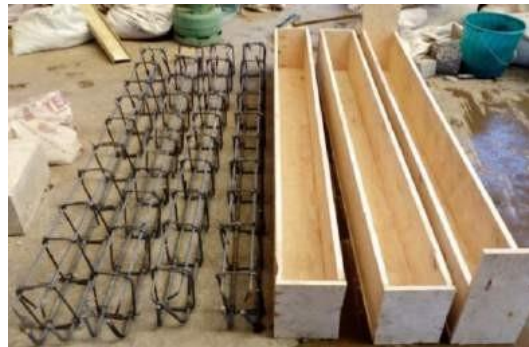
(a) Reinforcement details (b) Formwork and reinforcement cage Figure 2: Beam formwork and reinforcement details
