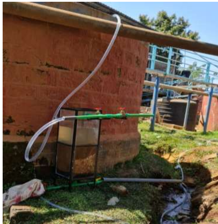
Model Filtration Unit Setup within an Existing Water Treatment Plant
