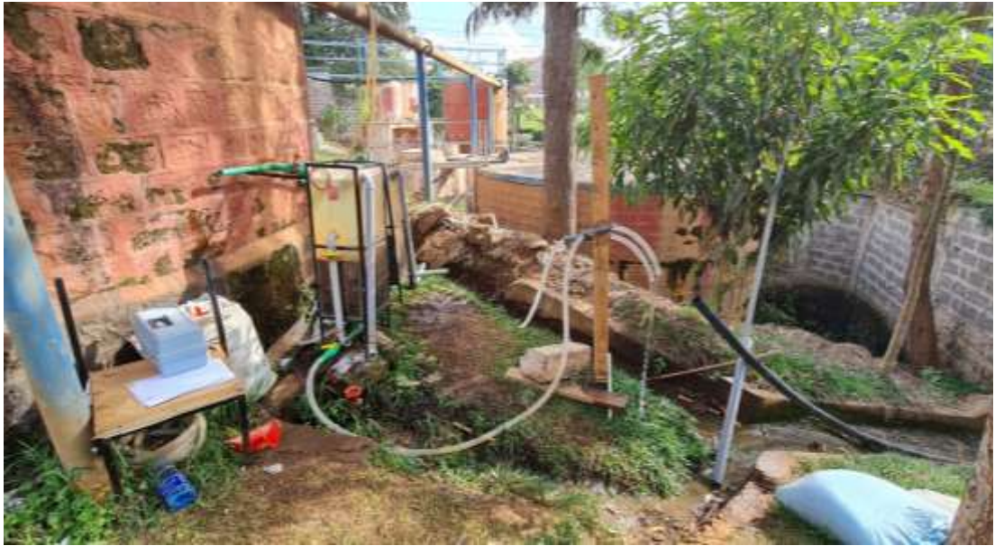
Ongoing Filtration Process
