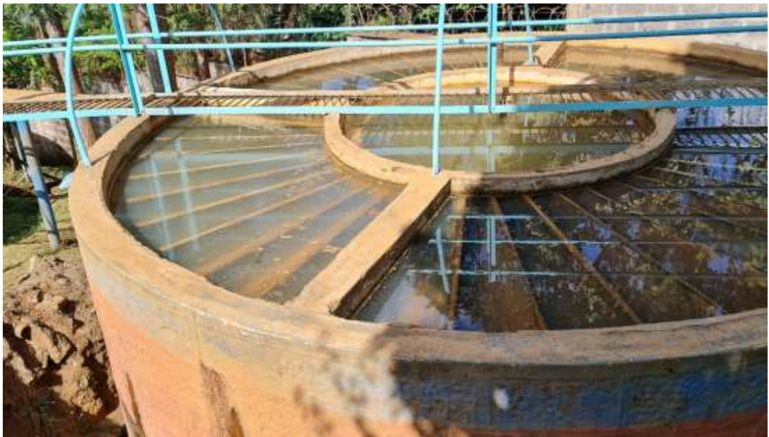
Pretreated Raw Water Source – Existing Clarifiers
