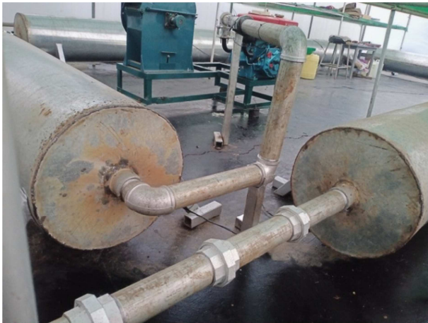
Figure 2. Recuperative heat exchanger in the solar-exhaust gas greenhouse dryer (reproduced from [35]).
