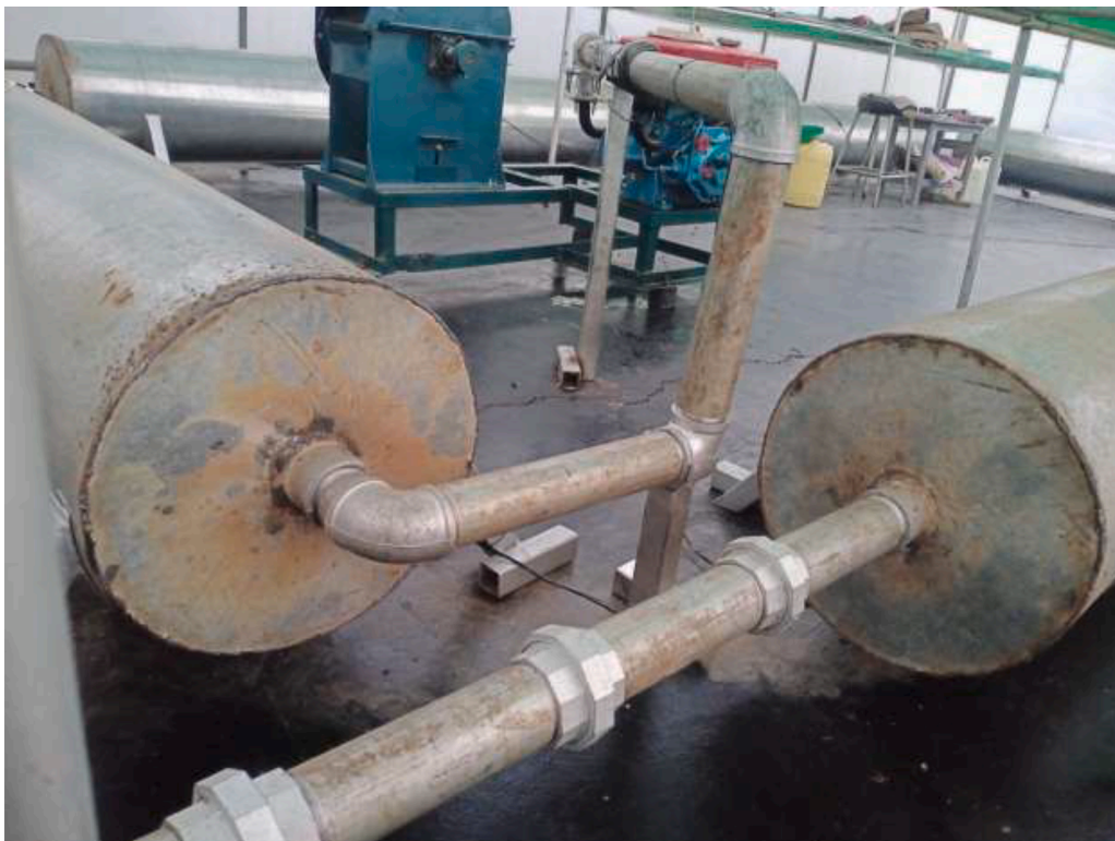
Fig. 2. Recuperative heat exchanger in the solar-exhaust gas greenhouse dryer.
