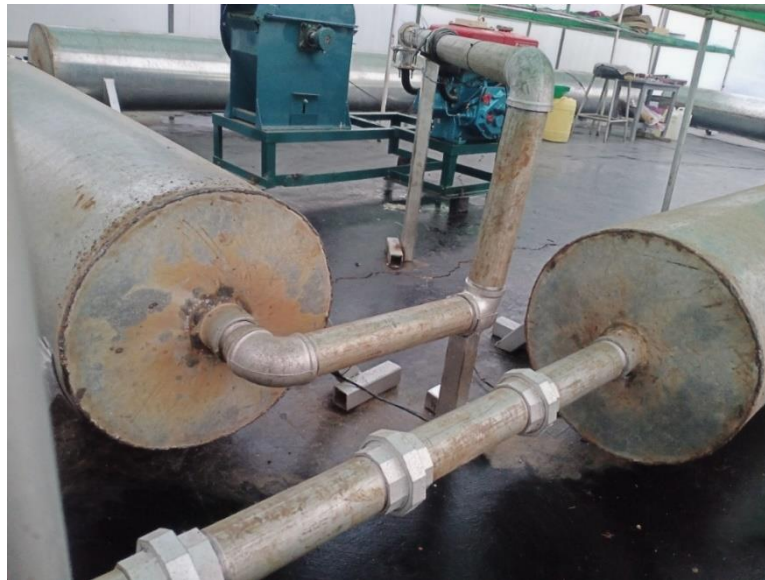
Plate B.2: Inside view of the solar-exhaust gas greenhouse dryer
