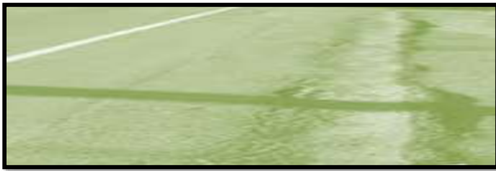
Figure 4.4: Rutting in Mombasa Road
