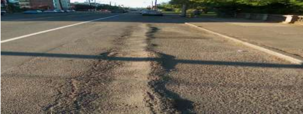
Figure 4.6: Ruttings and Cracks in Eastern Bypass
