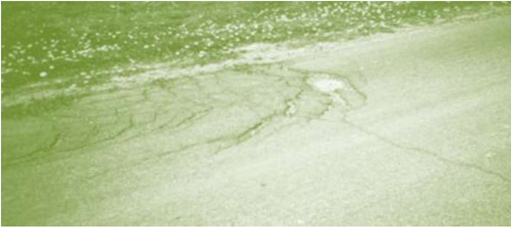
Figure 4.5: Potholes and Cracks along Mombasa Road
