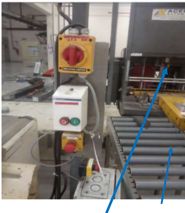
Plate 2.5: Isolators and E-Stops Fitted on Machines
