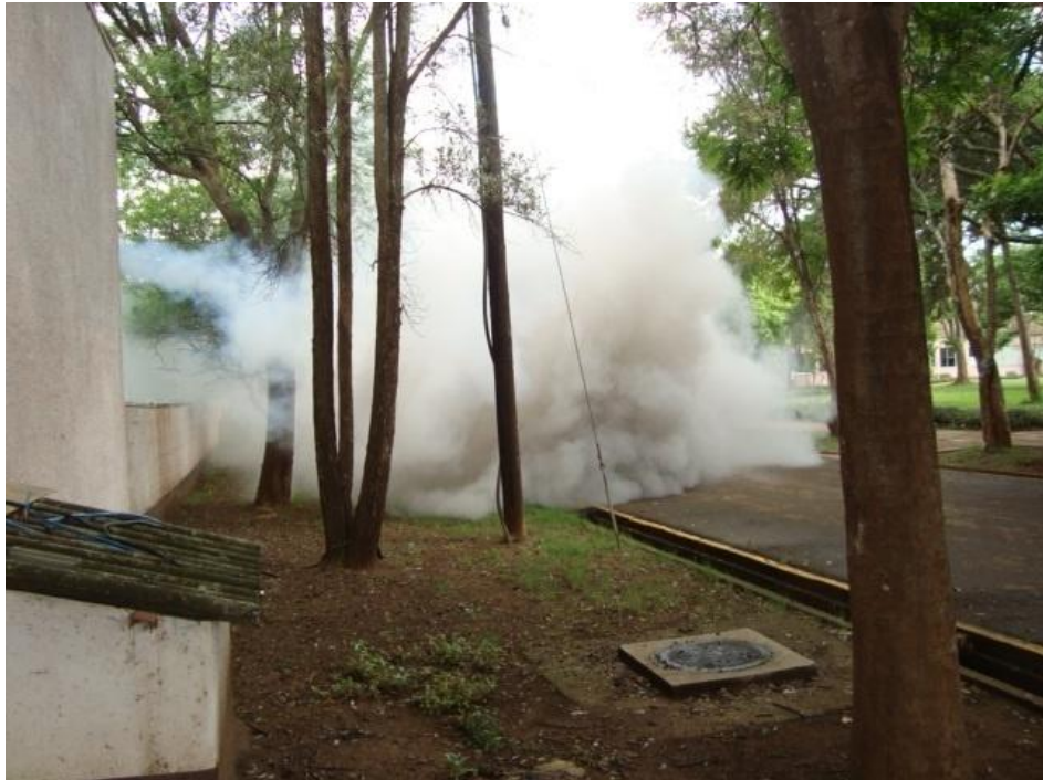
Plate 15 Dense smoke from the standby generator likely to block vision of road users on an adjacent road
