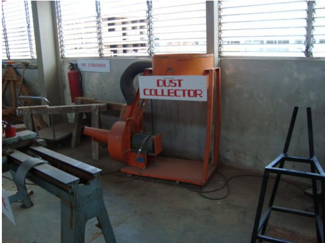
Plate 14 Dust extraction equipment in the carpentry workshop set aside due to lack of dust collection bags
