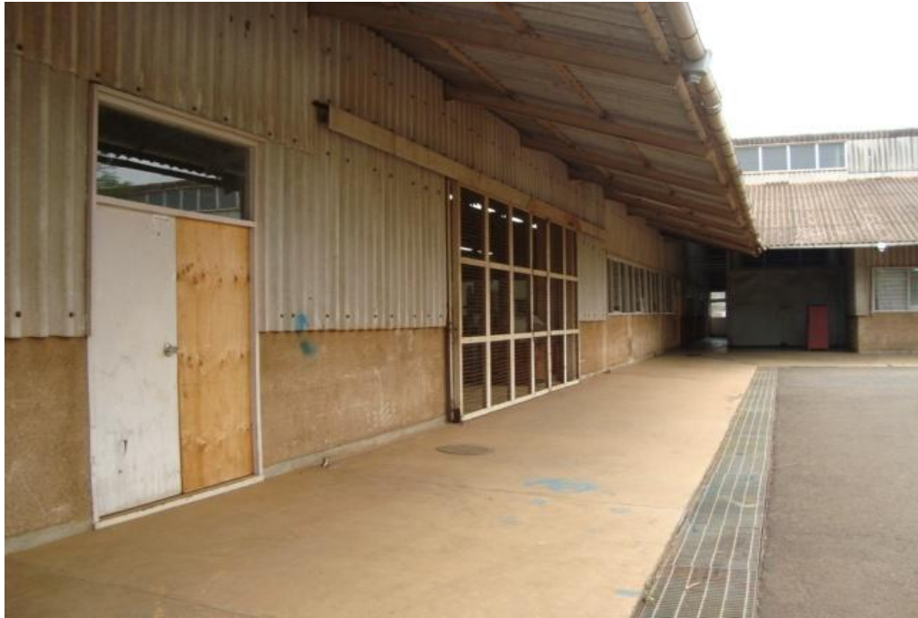
Plate 17 Asbestos cladding covering the Engineering Workshops likely to impart long-term adverse health effects to workers
