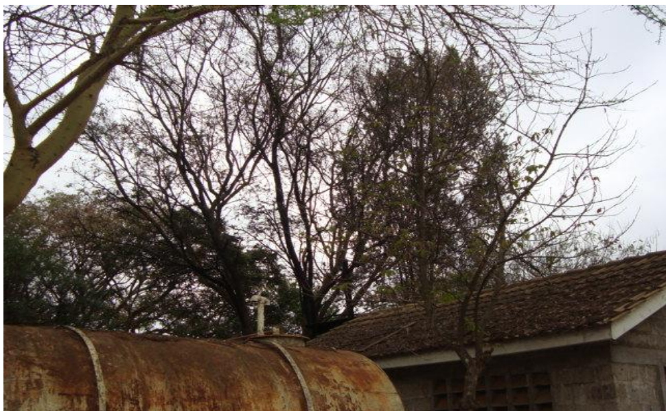
Plate 16 Adverse environmental effect of exhaust heat and fumes on vegetation and structures adjacent to the generator housing
