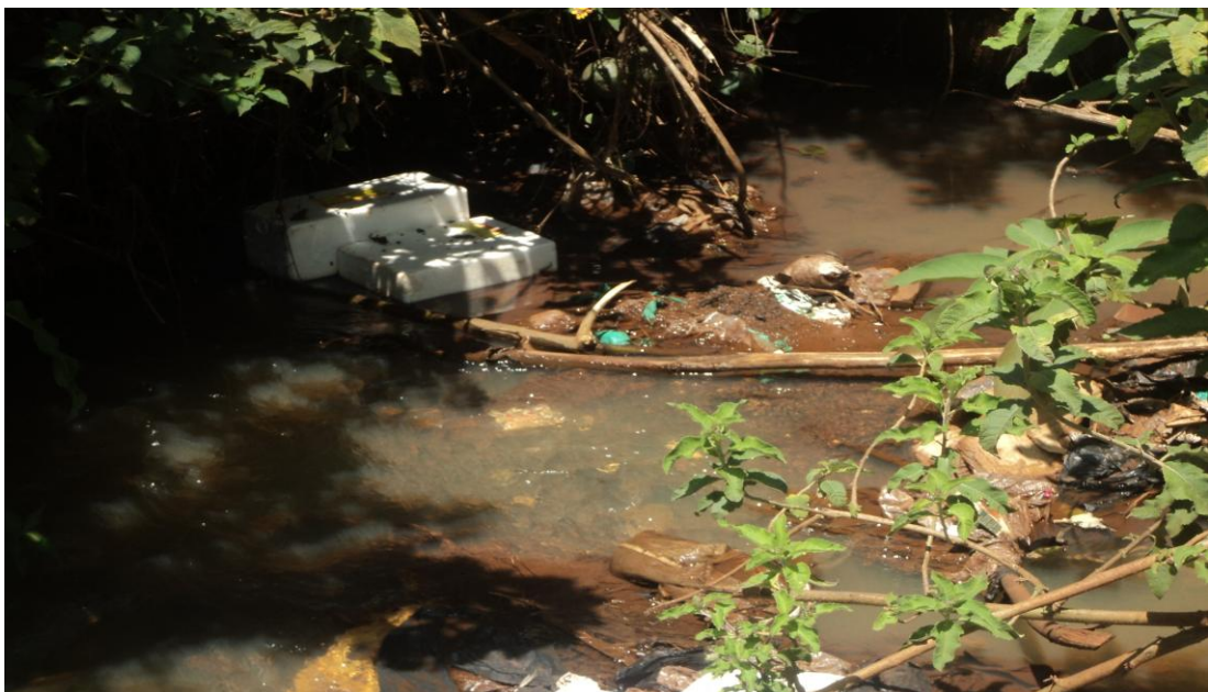
Plate 1.1: Clogged drainage due to solid wastes
